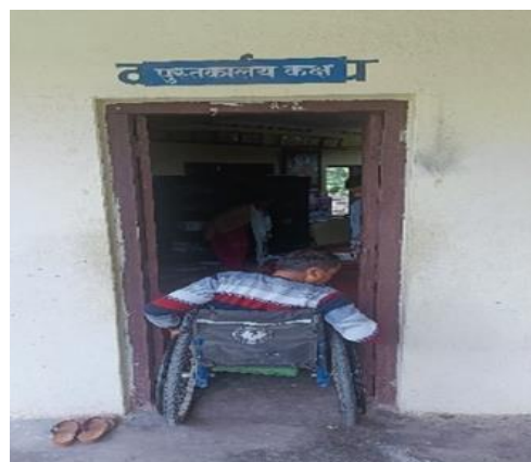
Insufficient width of door for wheel chair user
